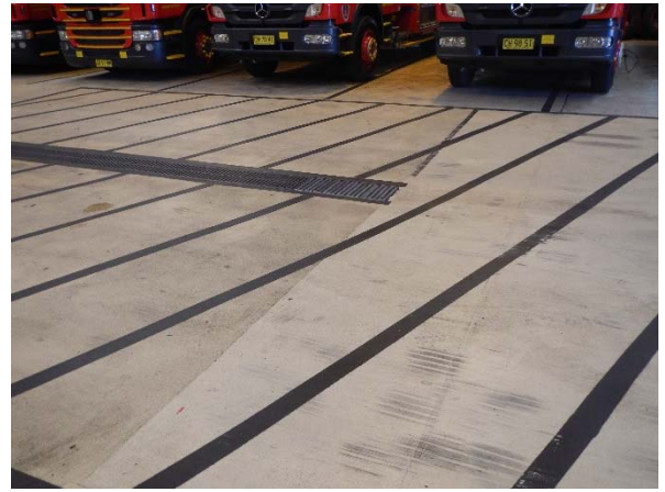
▲ Photograph 8: The building located in the north of the site that is used for mechanical maintenance and machine fit out with one internal drain located in the middle of the road..
