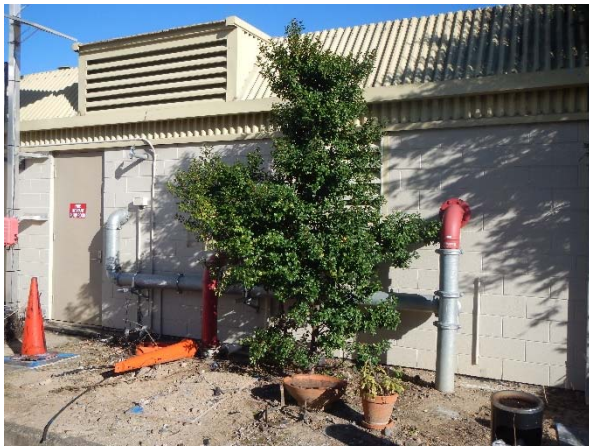
▲ Photograph 9: Generator for the site in the western area of the site.
