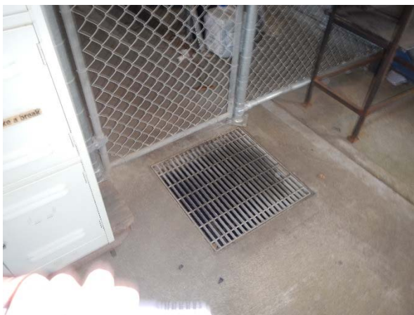
▲ Photograph 15: A drain outside the interceptor cage. Unsure if this is attached to the interceptor or stormwater for the site.
