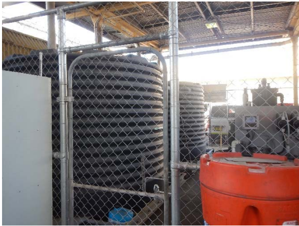
▲ Photograph 13: The interceptor and rain tanks located near the truck wash in the eastern area of the site.
