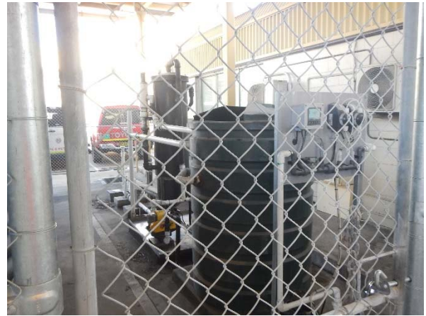
▲ Photograph 14: The interceptor for the site where the internal drains go to.
